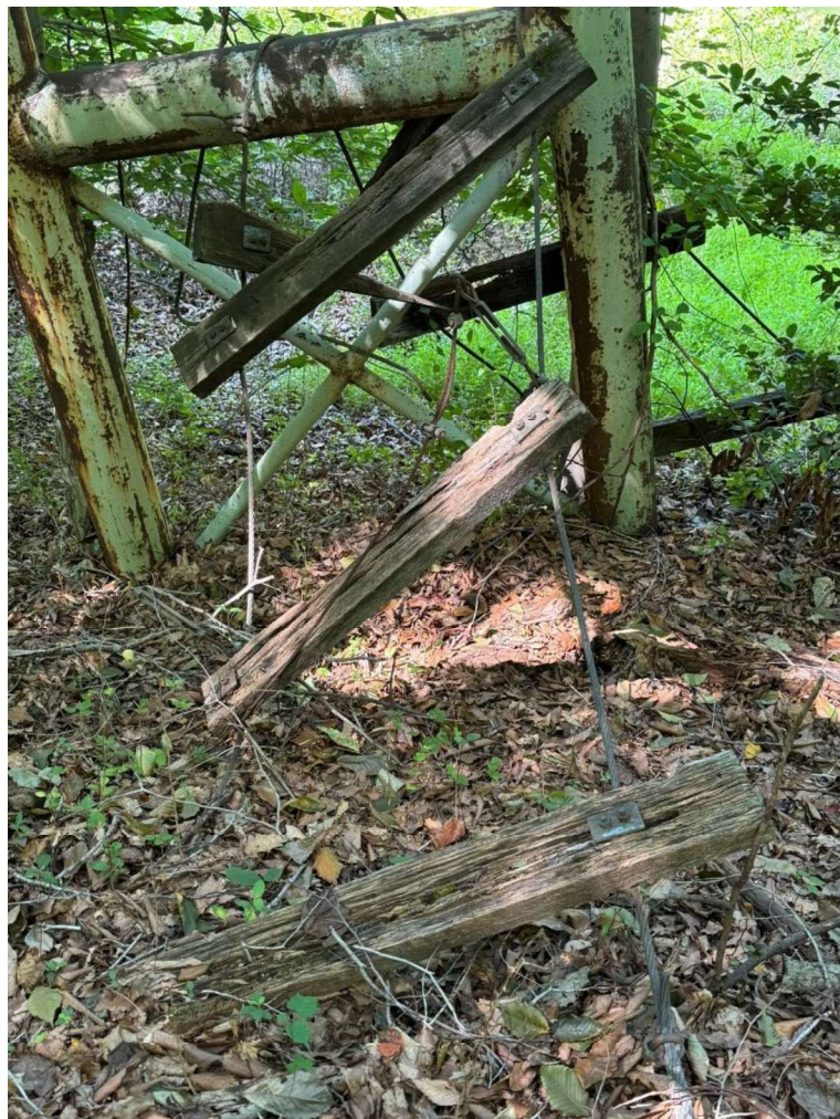
Figure 10 (Bottom) – Remains of a support for the Maryland Gas Transmission Company Swinging Bridge. Pieces of steel cable and foot-planks are still evident.
